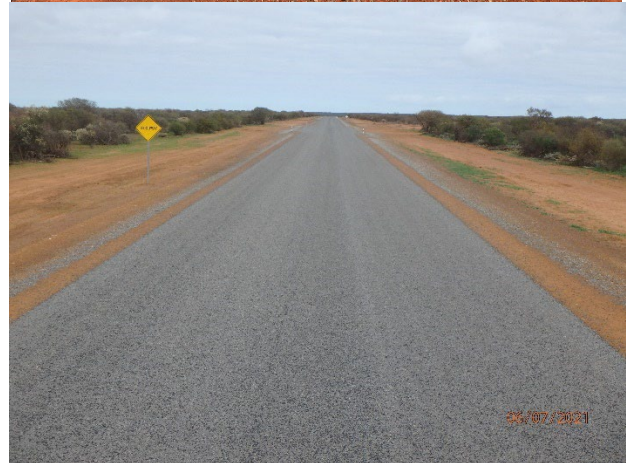
top to bottom left to right – Construction Crew, Two Pics Roadworks Construction Carnarvon-Mullewa Road, Ripping Works, Bituminous Sealing and finished result on Carnarvon-Mullewa Road.
